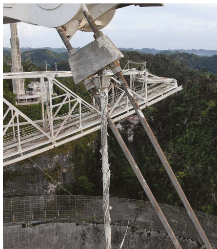
Broken wires on the second failed cable.
