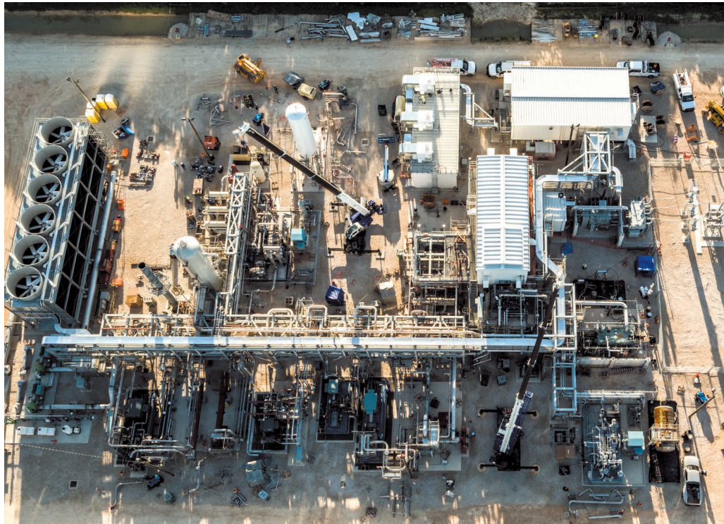
A demonstration power plant run by NET Power in Houston, Texas.
