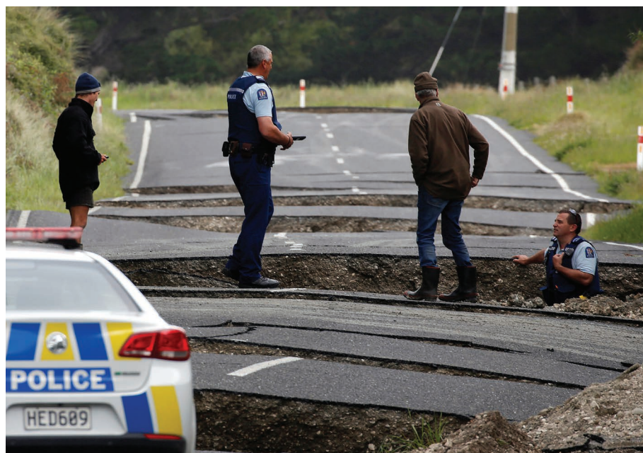
The Kaikoura earthquake in 2016 caused extensive damage on New Zealand's South Island.
